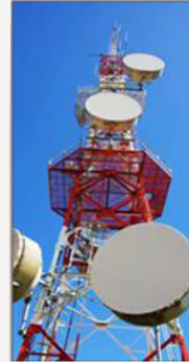
RADIO DEVICES AND TELECOM SHELTER
