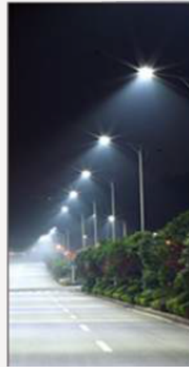
STREET LIGHTING AND PUBLIC UTILITIES
